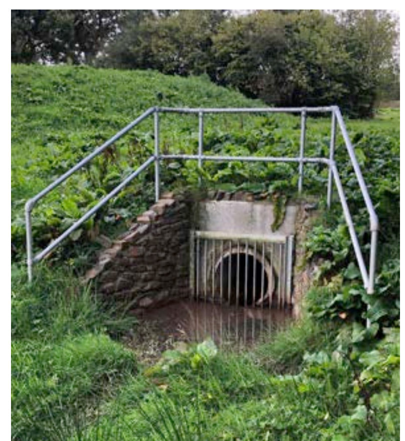
POTENTIAL TO INCLUDE MORE NATURAL HEADWALLS / INLETS AS PART OF THE SUDS TO INTEGRATE INTO LANDSCAPING
