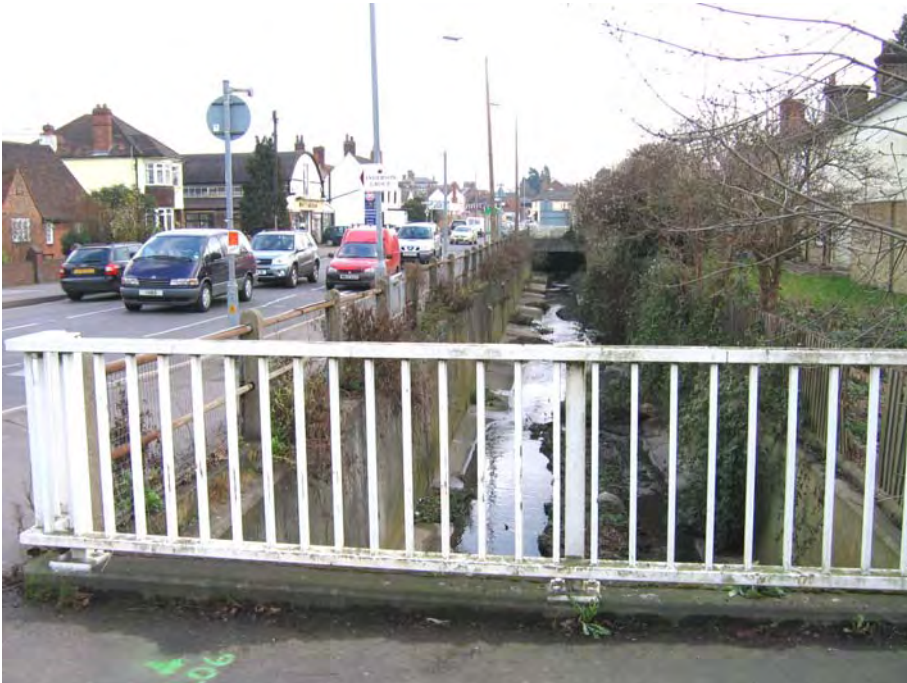
Fig. 36 West end of West Street, the concrete lined conduit for the Iron Well Stream.
