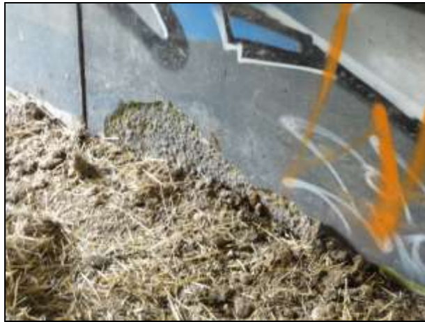
Photograph 16: Defect on south side of structure
