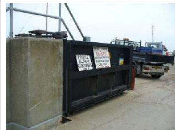
ROC04 Flood Gate at Paglesham.
