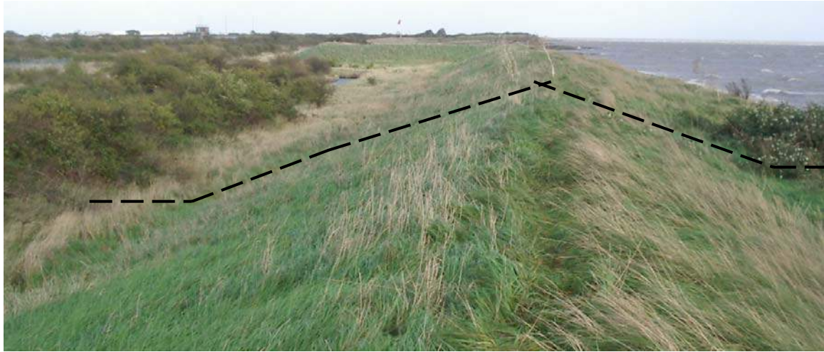
PLATE 6-1 A GRASSED EARTH BUND EXAMPLE ALONG THE NORTH SEA COASTLINE IN ROCHFORD
