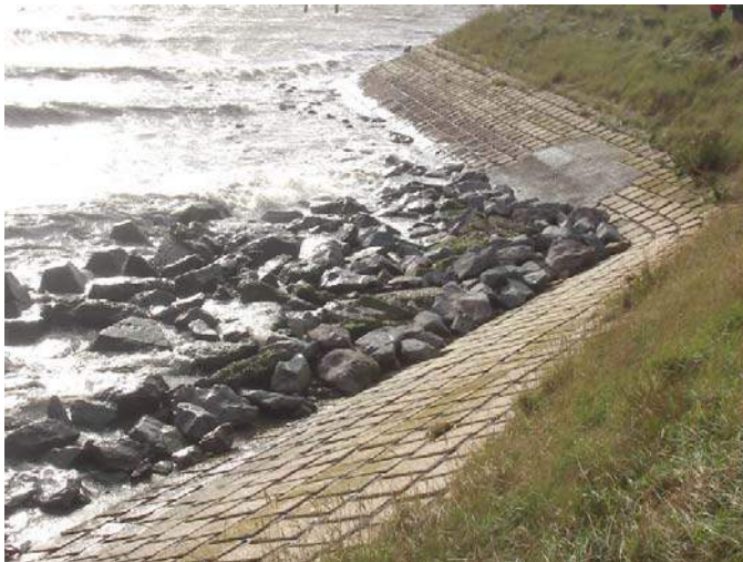
PLATE 6-3 ESSEX BLOCK REVETMENT ON AN EARTH BUND WITH ADDITIONAL ROCK ARMOUR TOE PROTECTION PROVIDING GREATER STABILITY AT THE TOE OF THE STRUCTURE, REDUCING UNDERCUTTING AND EROSION (SOUTHEND).
