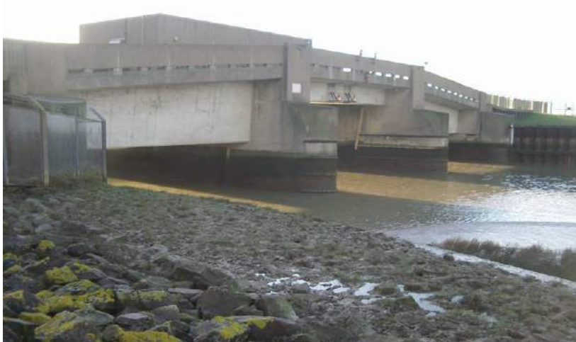
PLATE 6-11 EAST CREEK BARRIER ACROSS EAST HAVEN CREEK AT THE CONFLUENCE WITH HOLEHAVEN CREEK ON CANVEY ISLAND.
