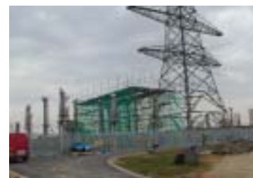
Sealing end compound.
