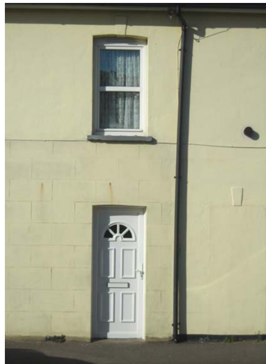
Fig. 79 Plastic replacement window and door, Prospect Cottages.
