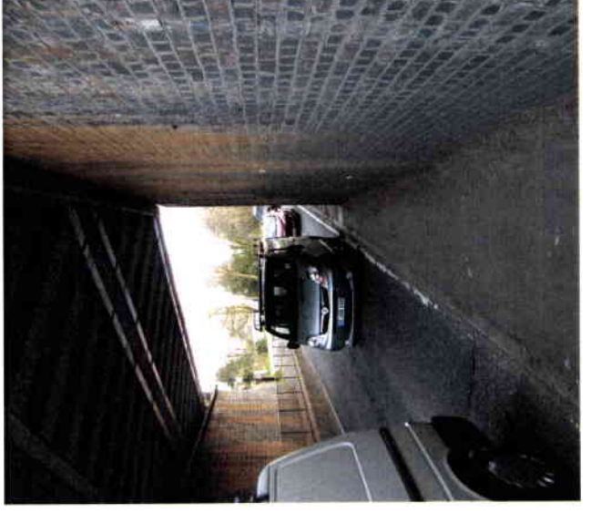
Photo 24: Physical limitation of railway bridge
