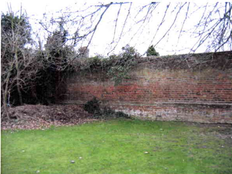
Fig. 18 Hall Road, one of the least overgrown parts of the Tudor boundary wall.
