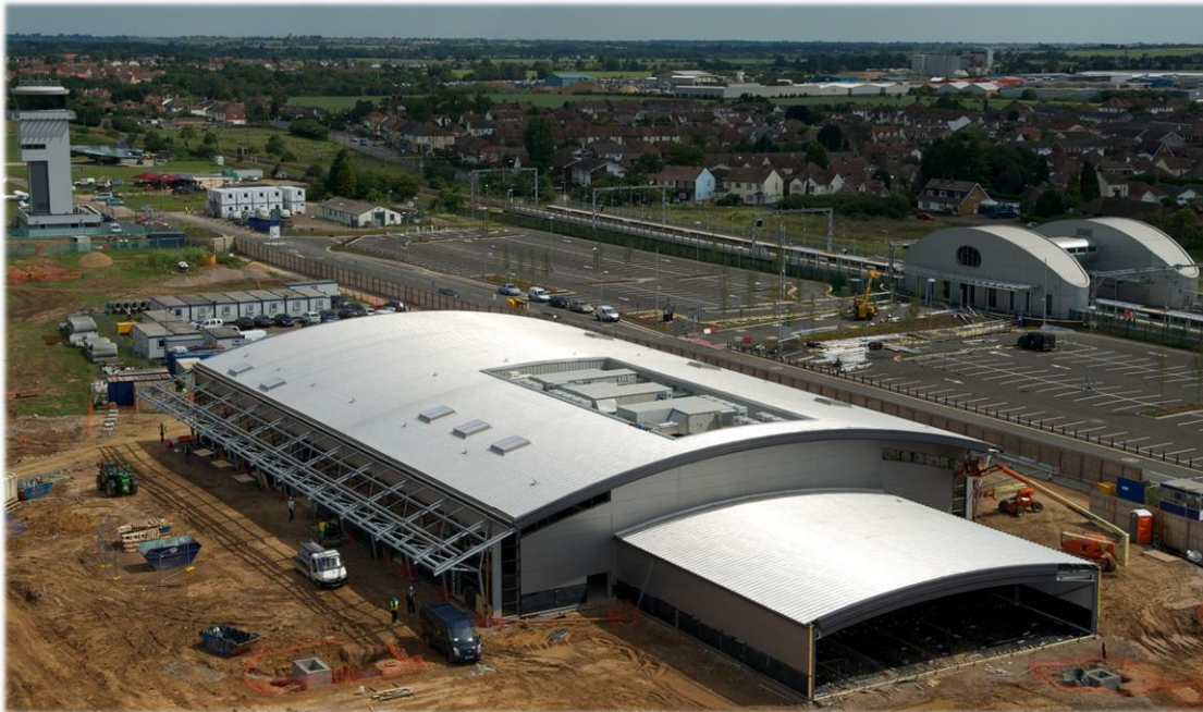
New passenger terminal, with control tower and rail station in the background
